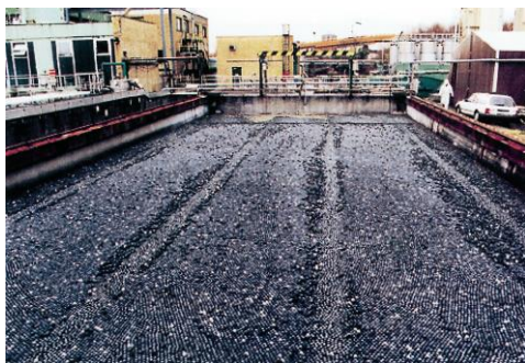
Black ALLPLAS balls, PP, Ø 70 mm, cover a rectangular tank with sweeper arm containing sewage water of an industrial chemical plant in Germany
