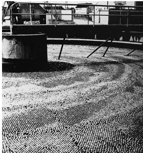
A layer of ALLPLAS balls covers a settling tank at a sewage treatment plant in Germany. Note that the balls automatically rearrange themselves around the moving support members of the sweeper arm. A single layer of ALLPLAS balls reduced odour generation at far less costs than conventional solid covers, yet satisfied the air quality demands of nearby residents.
