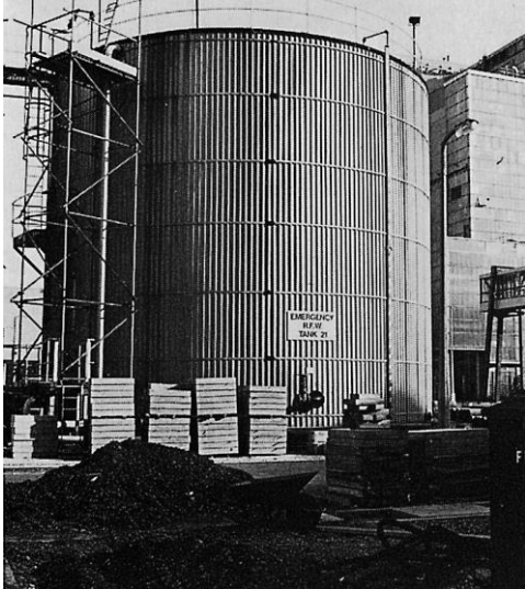
One of six condensate storage tanks at a British nuclear power station. The reactor containment buildings is in the background.
